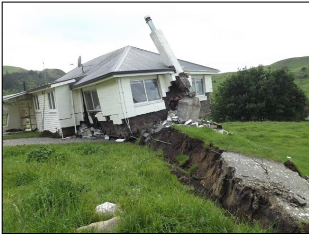
Figure 8: Direct fault surface rupture of c.8 m (dextral) through a farm worker's house across the Kekerengu Fault (Lat 41.978^{\circ}\text{S} , Lon 178.998^{\circ}\text{E} ; view to the west; photograph by Tim Little).
