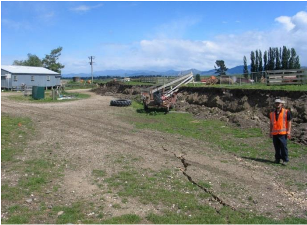
Figure 3: Oblique dip slip-dextral fault scarp of The Humps Fault at Glenbourne Farm that caused displacement damage to concrete slabs, farm tracks and fencing (Lat 42.615°S, Lon 173.105°E; view west; photograph by Jarg Pettinga).
