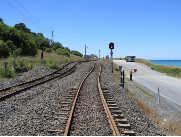
Figure 7: Dextral-reverse displacement of the SIMT and State Highway 1 across the Hundalee Fault at Oaro (Lat 42.504^{\circ}\text{S} , Lon 173.510^{\circ}\text{E} ). The displacement of the road was sharp, but smoothing and resurfacing was just being completed when the photo was taken. The SIMT offset was diffused through embankment ballast and the flexibility of the rails, and in this view has yet to undergo any repair or modification (photograph by Mark Stirling).
