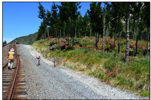
Figure 11: Surface fault rupture across a northeastern strand of the Papatea Fault near the coast deformed and distorted the SIMT line and severed the East Coast fibre optic cable at this location. Orange flagging marks the location where the fibre optic cable was cut by fault rupture and subsequently repaired (view to the southwest; photograph by Robert Zinke).
