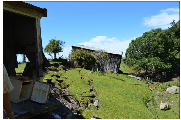
Figure 10: Rupture through farm buildings on a southwestern stand of the Papatea Fault near the coast (Lat 42.201^{\circ}\text{S} , Lon 173.875^{\circ}\text{E} ; view to the south; photograph by Robert Zinke).
